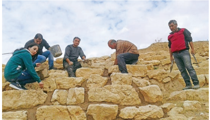
Figure 1. Conservation work on the monumental staircase of the Great Temple of Urkesh in Tell Mozan takes place every fall in preparation for winter. This image, taken in October 2015, shows local men and women placing fresh mud mortar to protect the joints between stones.
