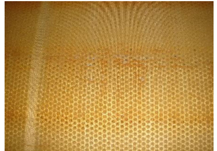
BaSO 4 scale choking washer wire holes
