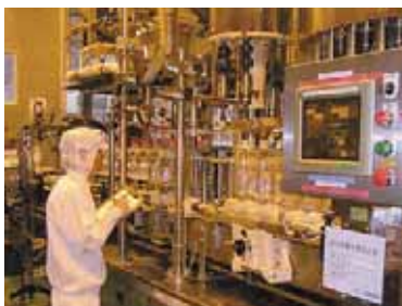
Filling facilities in a clean room
