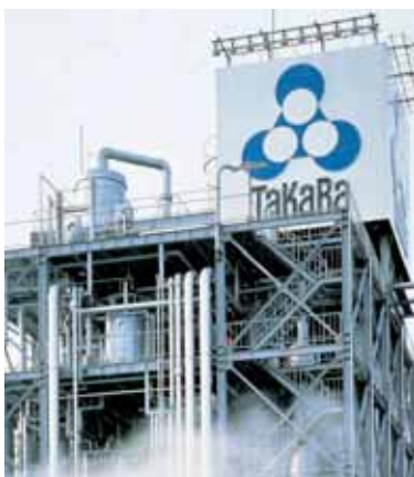
Continuous distillation equipment
