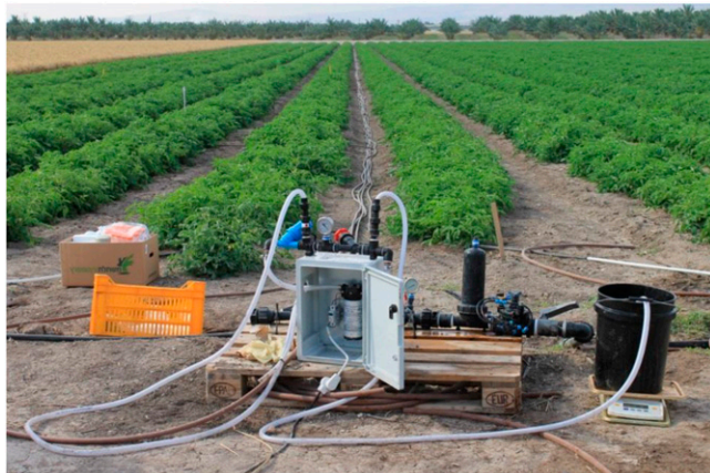
Fig. 10. Electric pump setup for injection of herbicides into drip line systems in field experiments.
