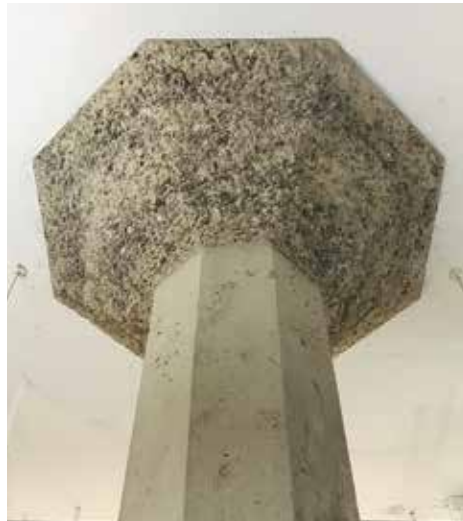
Architects from Salt Lake-based Blalock & Partners stripped the interior to its historic roots, uncovering an old brick wall with great character and utilizing this unique concrete column with an exposed aggregate column cap.
