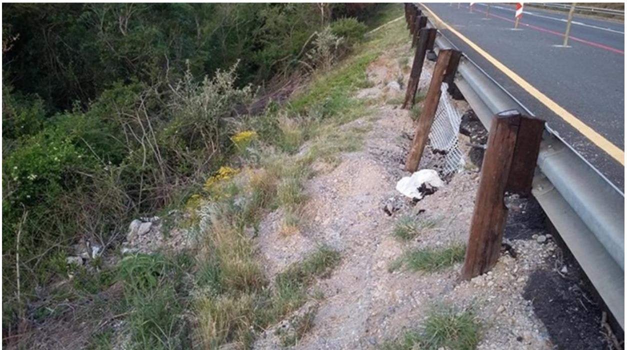
Figure 3: Gaps in the existing bitumen pre-mix curbs and resultant erosion and slumping down the embankment at approximate chainage km 43.130
