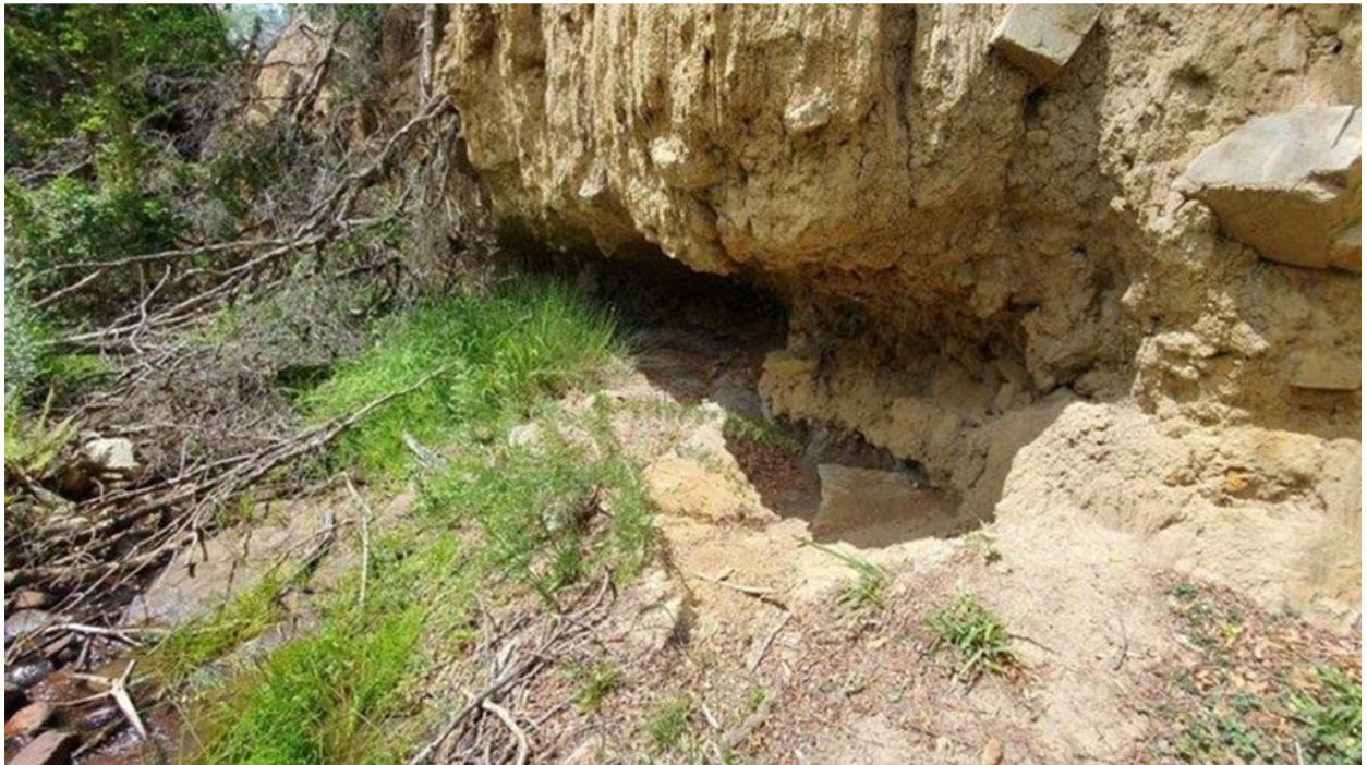
Figure 2: Undercut embankment along the Berg river at about chainage km 43.300.
