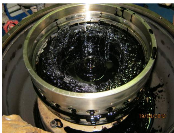
Figure 17 - excess sludge build up in the purifier bowl
