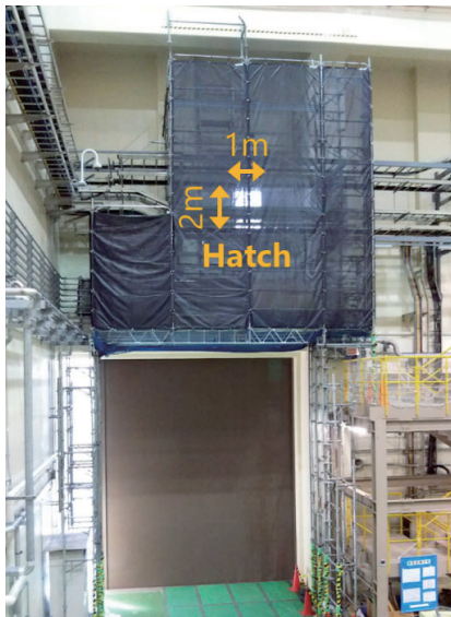
Figure 3. Aperture for electric transmission lines. It is located above the carry-in entrance of the east #1 experimental hall of the MLF.
