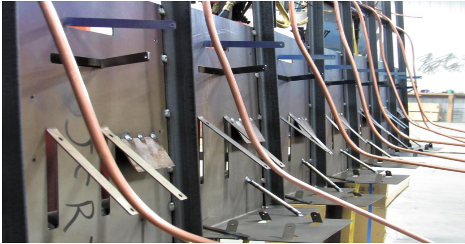
Units prepped for compressors
