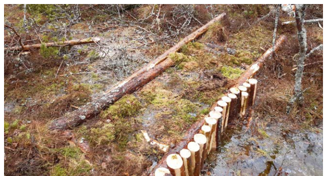
The framework for a dam made of birch trunks has been covered with peat. Photo: Henri Jokinen.
