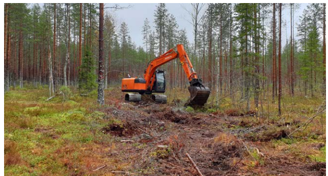
An excavator blocking a ditch in a mire.
