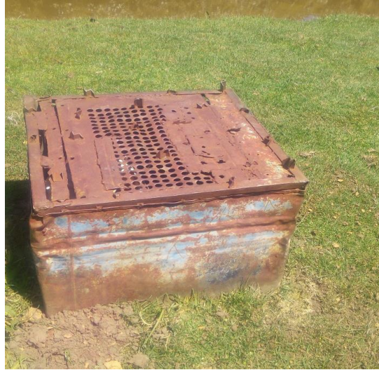
Plate 10: Water pump housing: for pumping water from wetland
