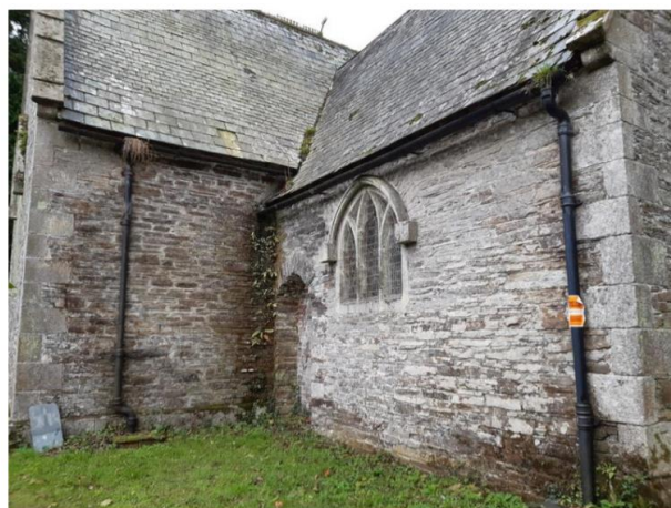
View of church from north east showing the east facing wall of the northern transept and the north facing wall of the chancel.
