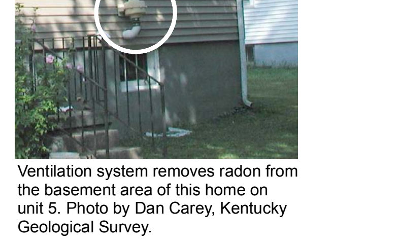
Ventilation system removes radon from the basement area of this home on unit 53. Photo by Dan Carey, Kentucky Geological Survey.
