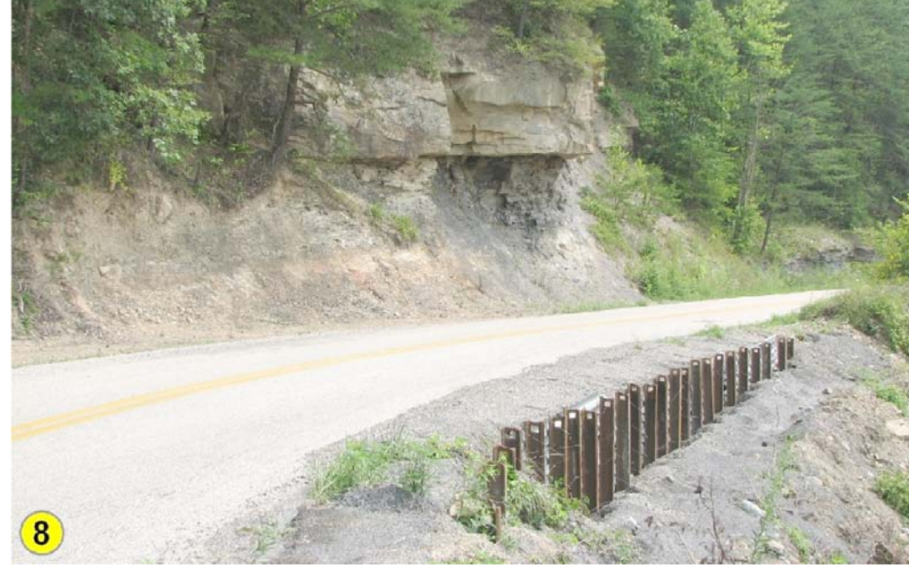
Sandstone and siltstone overlie shale of unit 5 along Ky. 3333. The roadbed support is typical of that used to prevent pavement failure for roads built on shale. Photo by Dan Carey, Kentucky Geological Survey.
