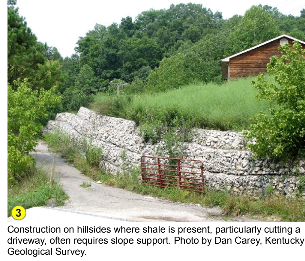
Construction on hillsides where shale is present, particularly cutting a driveway, often requires slope support. Photo by Dan Carey, Kentucky Geological Survey.
