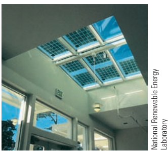
Rooftop solar cells may replace centralized power in the future.
