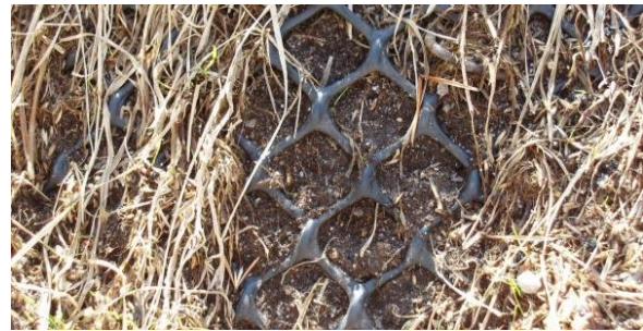
Permanent plastic lattice
