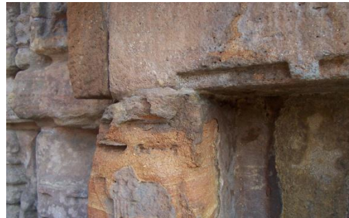
Figure 2 Salt efflorescence causing exfoliation and exposed pulverization of stone structure.
