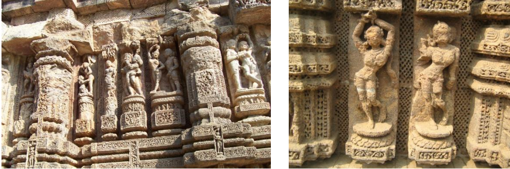
Figure 11 & 12 Abrasive action of the air borne salt particles striking especially at the higher portion of the temple structure.
