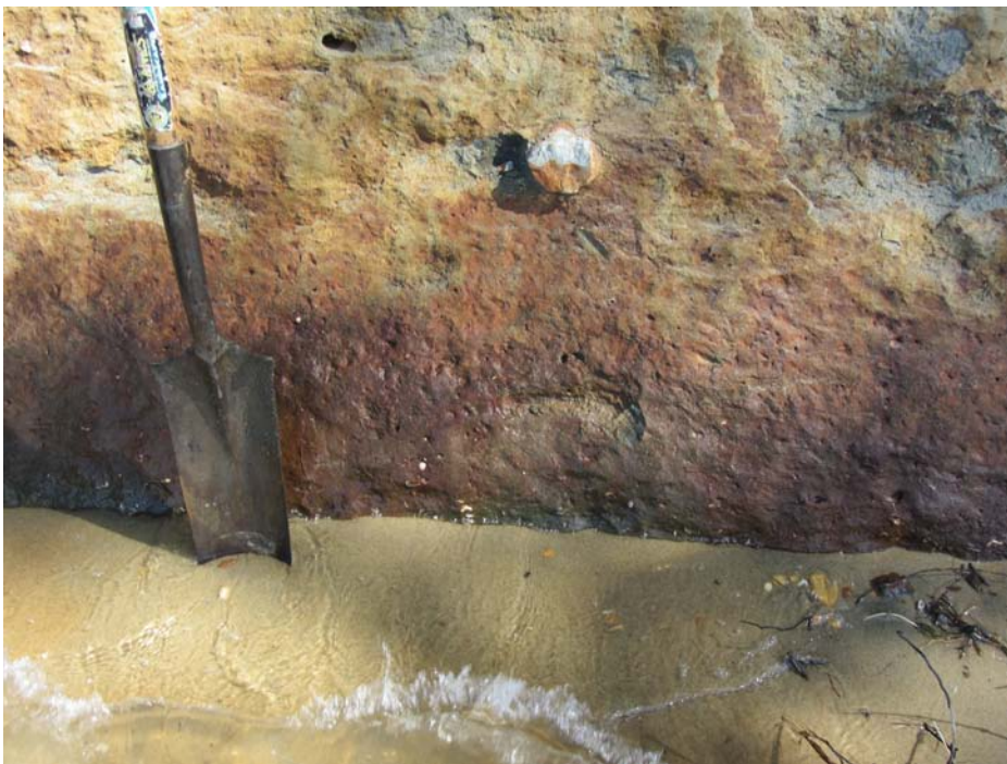
A close-up of the “splash zone”. The iron oxides occur only on the face. The round object that protrudes from the cliff face in the lateral middle of the photo, but close to the top vertically, is silica cemented. Sandy soil material of the beach lies against the bottom of the
