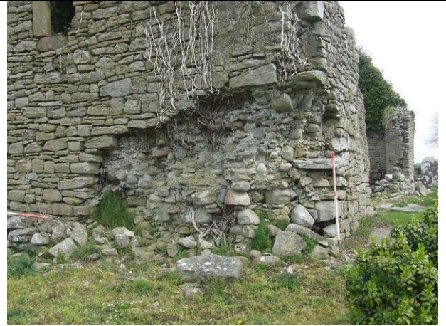
Plate 2 Showing west gable (southern end) prior to repair works, facing east.
