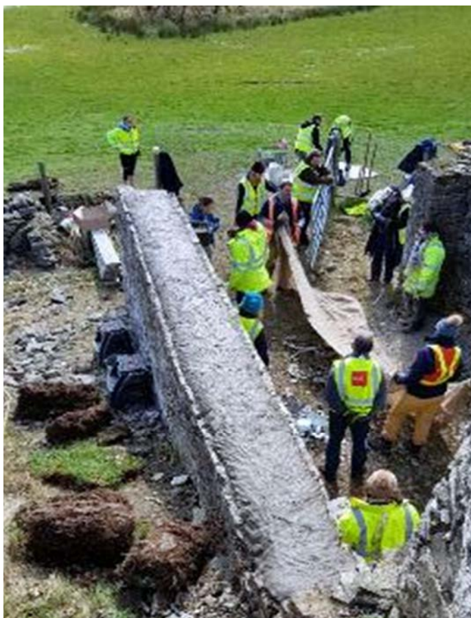
Example of soft cappings detail to stone walls, clay layer installed prior to laying sod.
