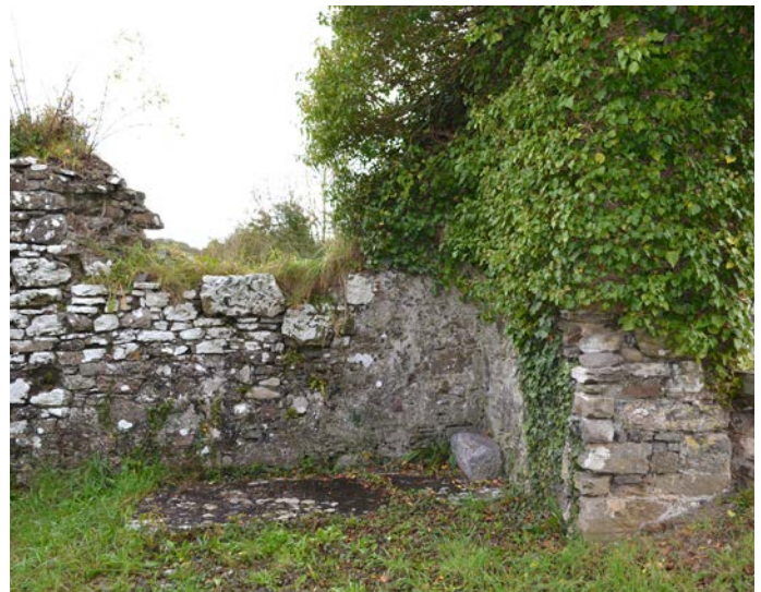
Corner of nave where north wall meets east gable, section of lime plaster still intact.
