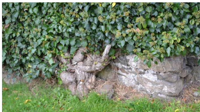
Typical ivy root on south wall.
