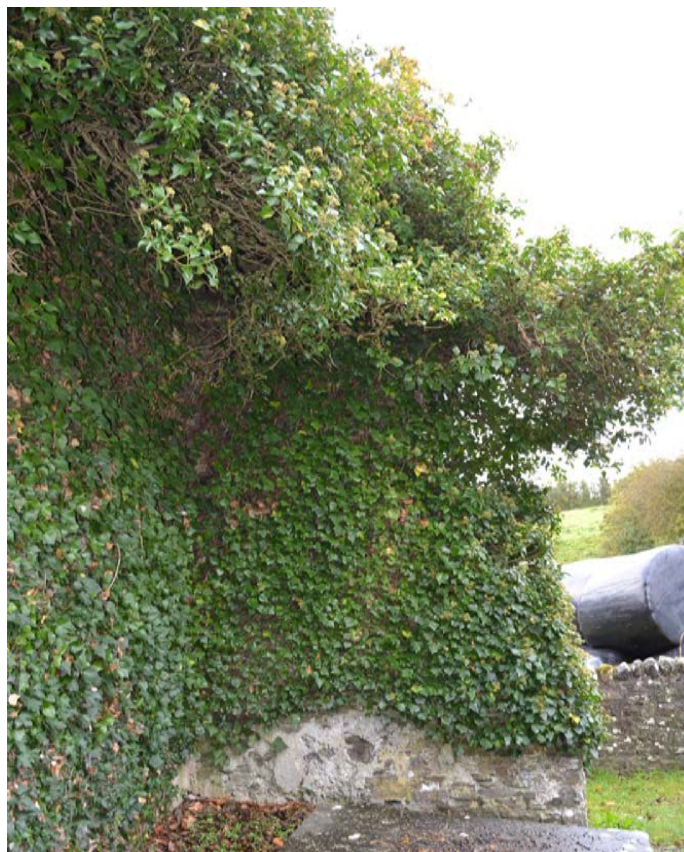
Prolific ivy growth on the church ruins that threatens the structural stability of the building. Image taken before trimming.
