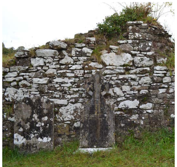
Detail of exposed masonry on the north wall of nave. Headstones laid against the nave wall.
