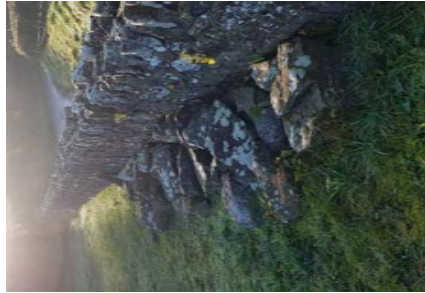
Fallen stone stored on site available for repairs
