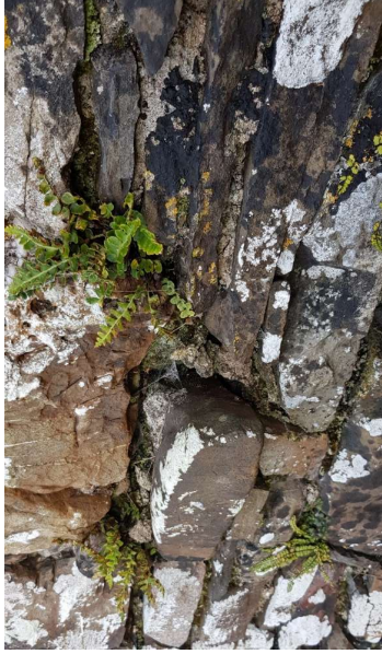
Vegetation growth with shallow roots on wall face, not harmful to wall
