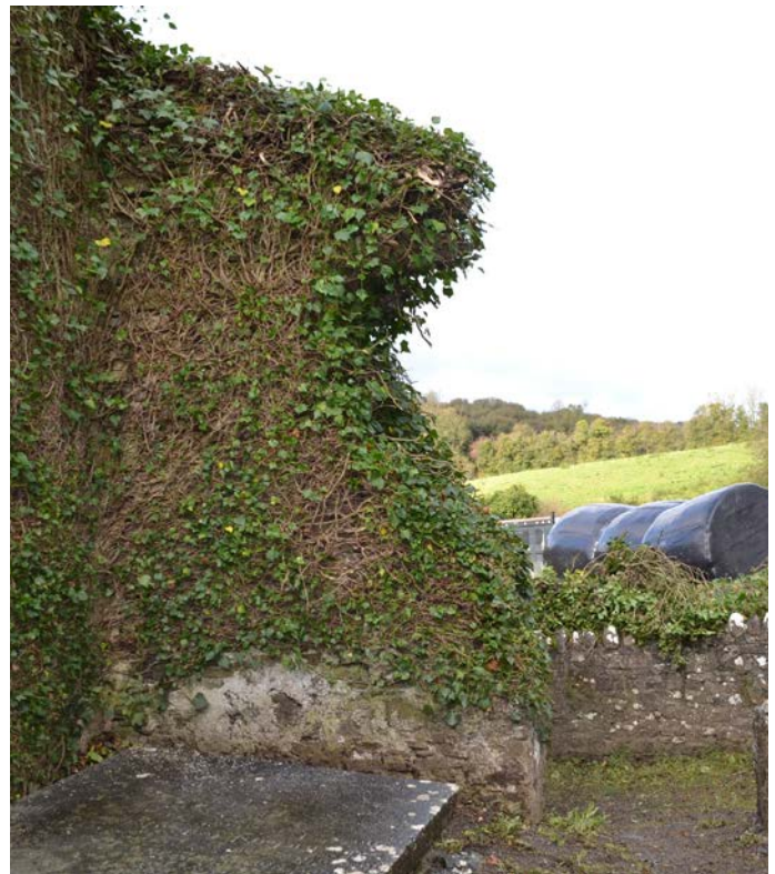
Loose masonry above north door.
