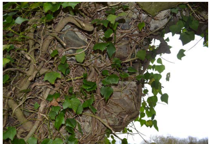
Loose masonry in arch of west window.
