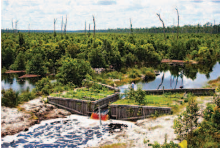
Figure 3: Dam constructed to systematically block a former logging canal to restore peat swamp water levels.
