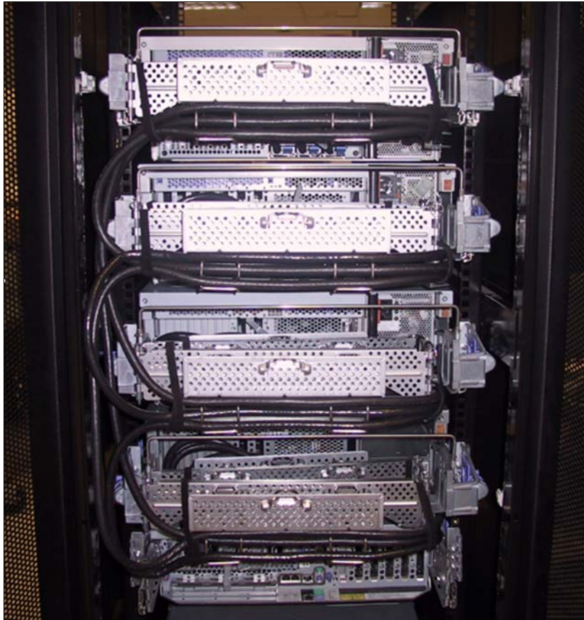
Figure 4-17 x3950 M2: four-node scalability cabling
