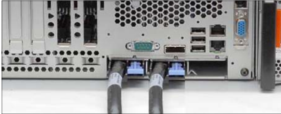
Figure 4-12 x3950 M2 - connected scalability cables
