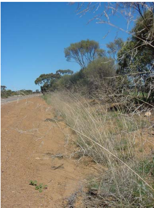
African lovegrass 'bunches' under the grader blade, requiring extra runs to remove it.
