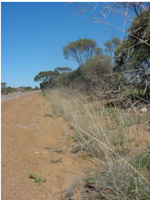
African Lovegrass is a perennial grass growing to 1.5 metres. It is common on road shoulders and in drains and can undermine the road structure.
