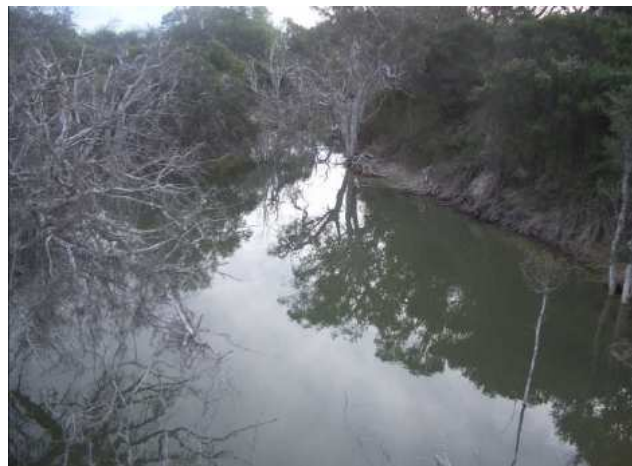
Plate 2. Standing water upstream of the Culvert Structure on Coolgardie-Esperance Highway
