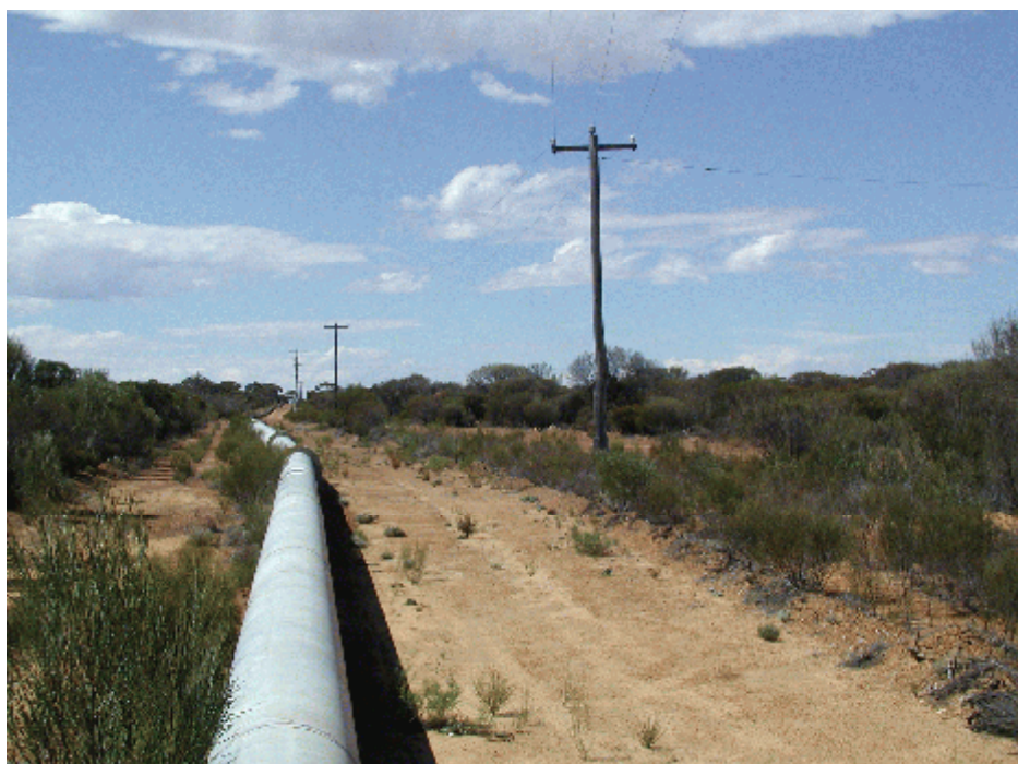
Figure 19: Power lines and the water pipeline between Coolgardie and Southern Cross.
