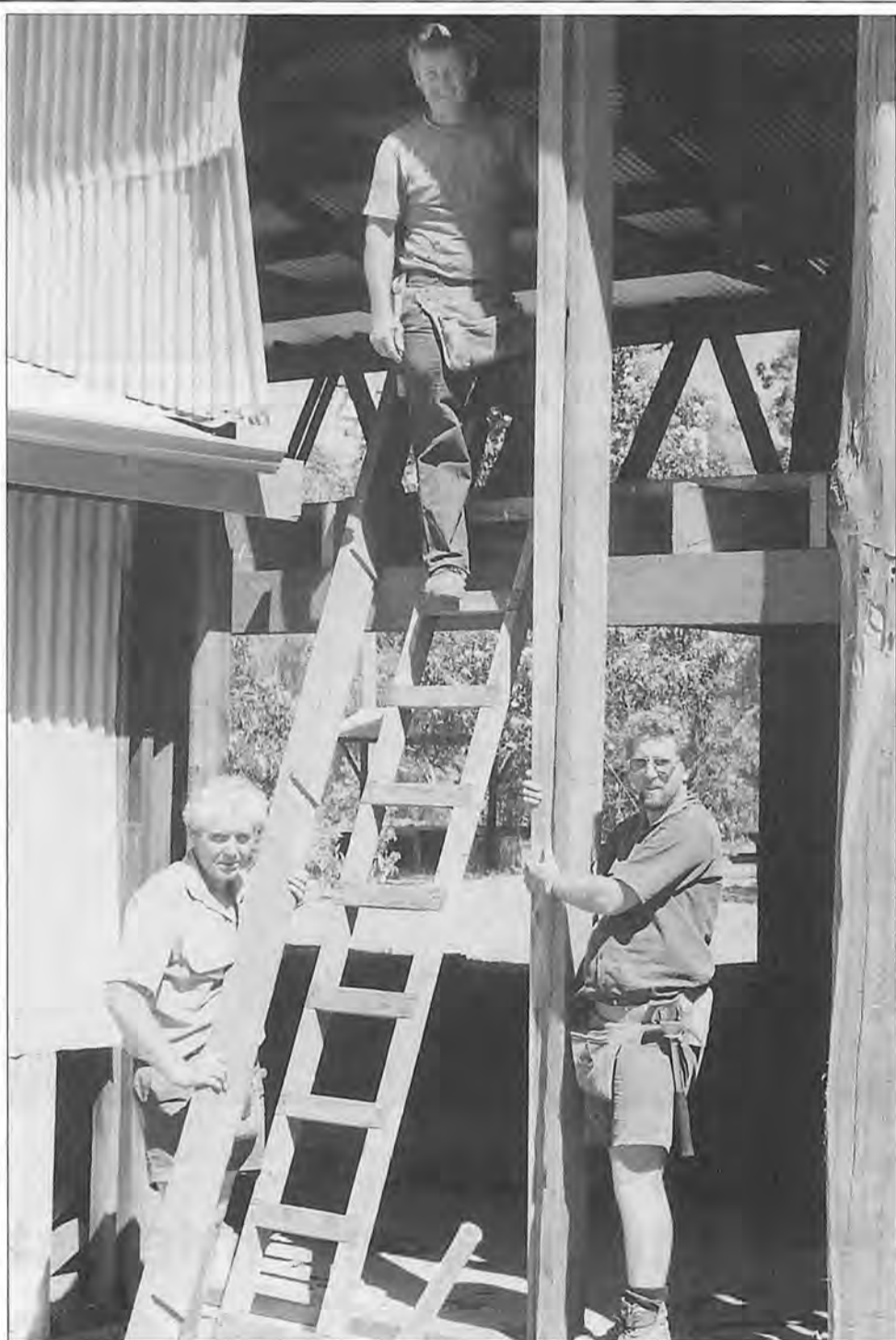
From left, CALM carpenters Toni King, Ray Bridges and Ken Howes during construction of bunkhouse. Photo by Glenn Willmott
