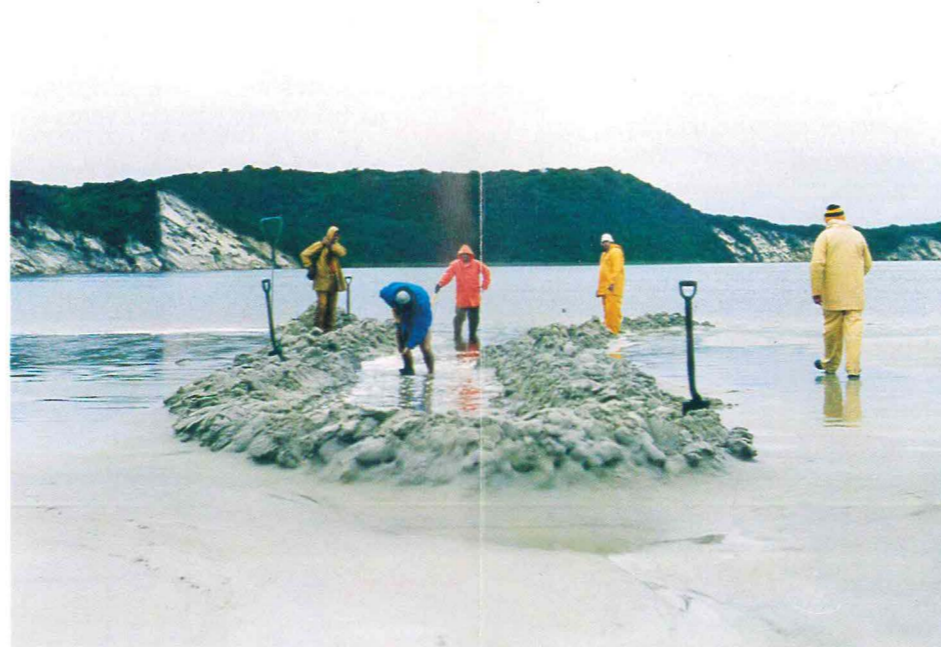
Irwin Inlet. Digging the cut through the bar, 31 May 1988 (Photo B. Gallash).
