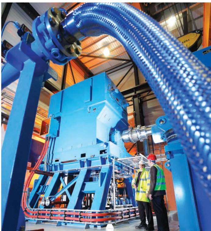
ABB's 3,256 kW water-cooled motoring.
