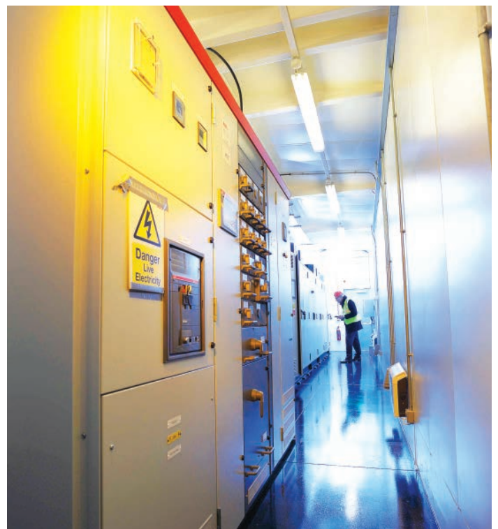
ABB supplied low and medium voltage switch gear.
