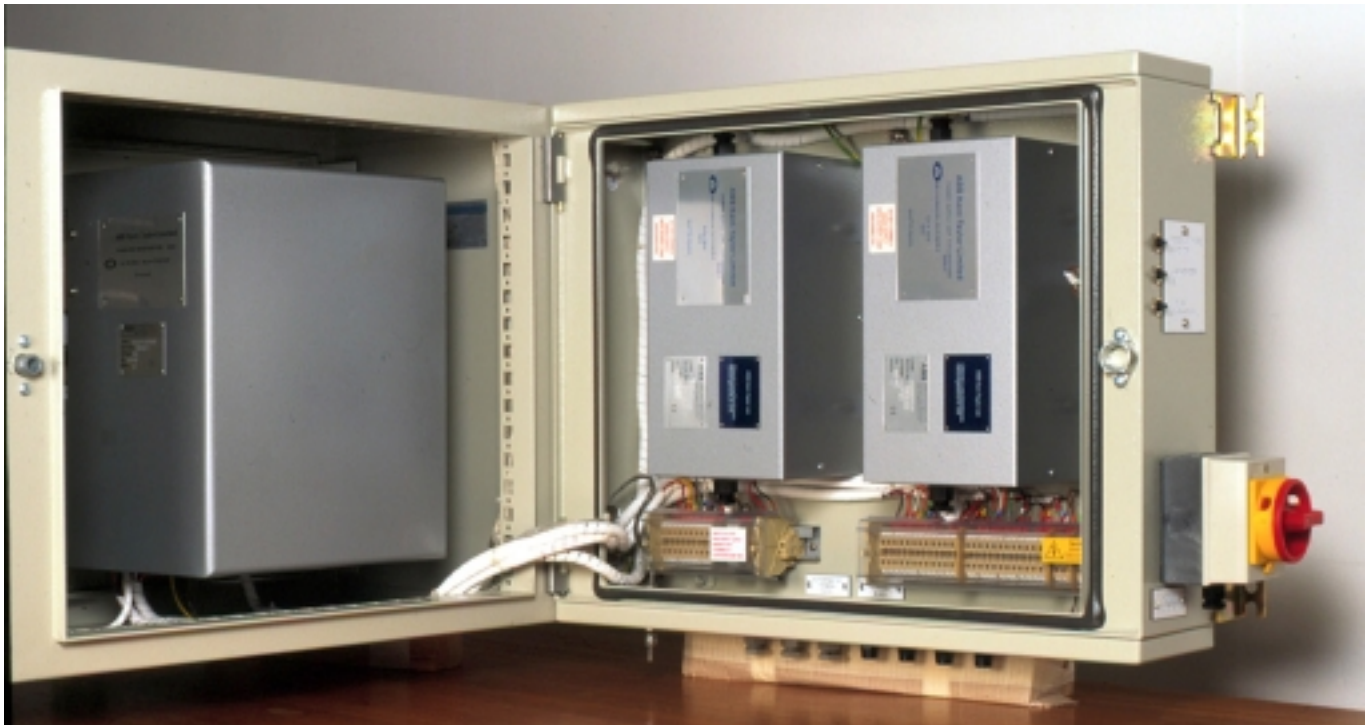
Rear View of Cubicle
