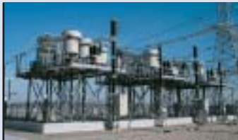
Flexible AC transmission systems (FACTS) enhance the capacity of existing networks and increase power quality. ABB has more than 600 FACTS installations, or 50 percent of the world market.
