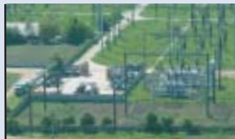
Transmission substations are used to raise voltages for long-distance power transmission. ABB has built more transmission and distribution substations than any other company – well over 5,000.
