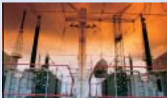
ABB power solutions deliver electricity from the grid to systems throughout the mill, and manage on-site generation of primary or backup power.
