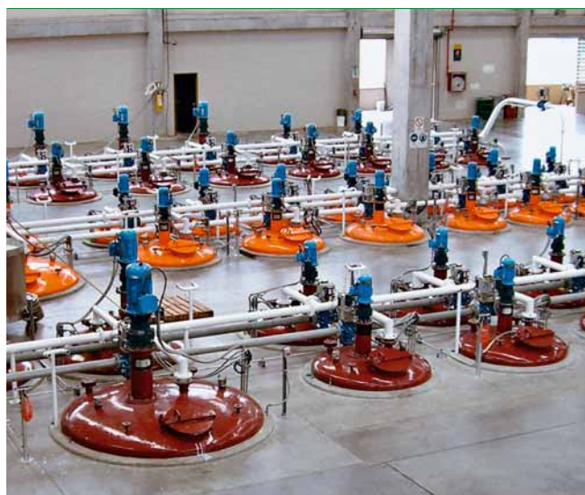
6 Piggable lines installed in the Pintuco paint manufacturing plant in Colombia
