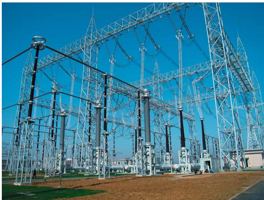
7 The 1,100 kV GIS substation Jingmen, China
