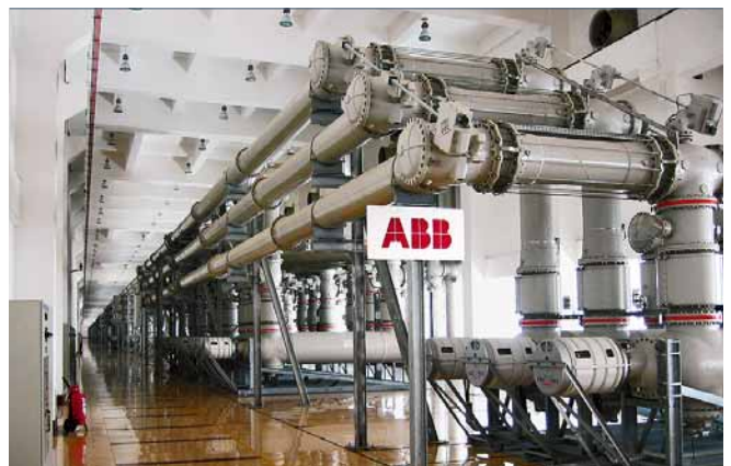
5 A 550 kV substation with GIS (rated at 550 kV, 63 kA, 4,000 A) installed within the dam at Three Gorges hydroelectric power plant in China
