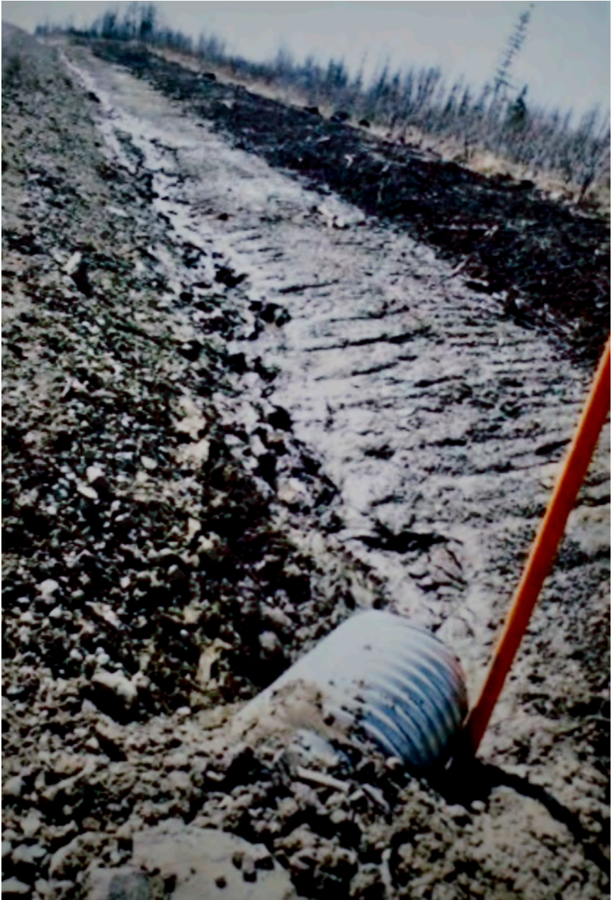
FIGURE 9.6. Flow Gauge Installation on the Brassy Creek. Photo by Reg Whiten.
