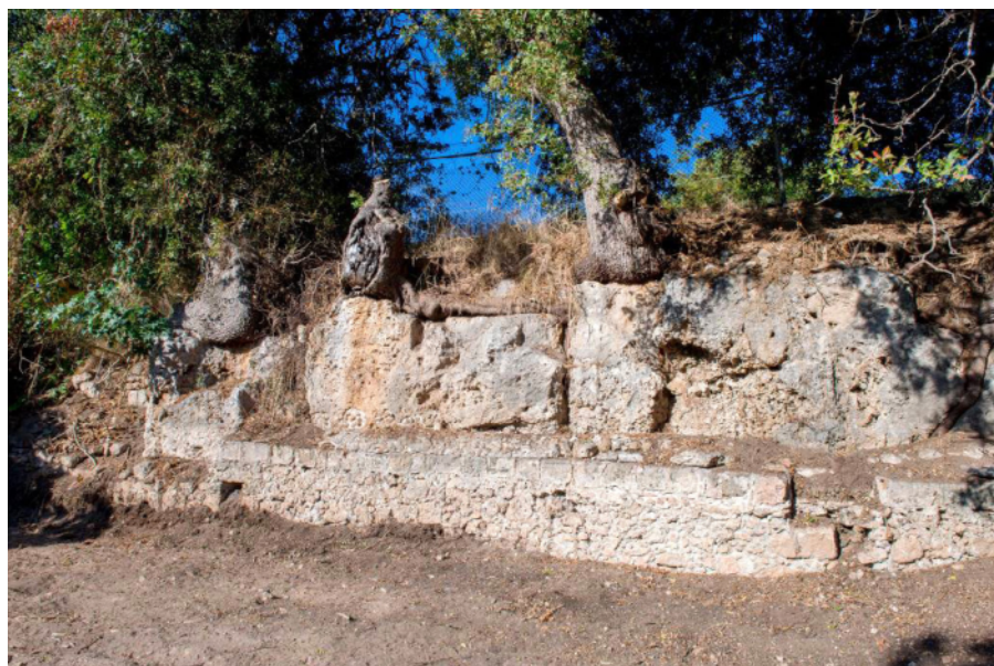
Figure 13. Clearing works 2017. Rock terrace wall on the southeast slope of the hill.
