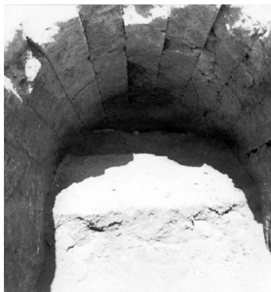
Figure 6. The vaulted ceiling of the staircase leading to the subterranean water system.
