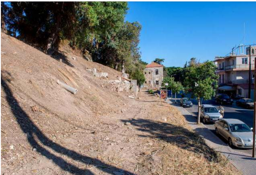
Figure 12. Clearing works in 2017. The east slope of the hill along M. Konstantinou Street, the ancient street P 30.
