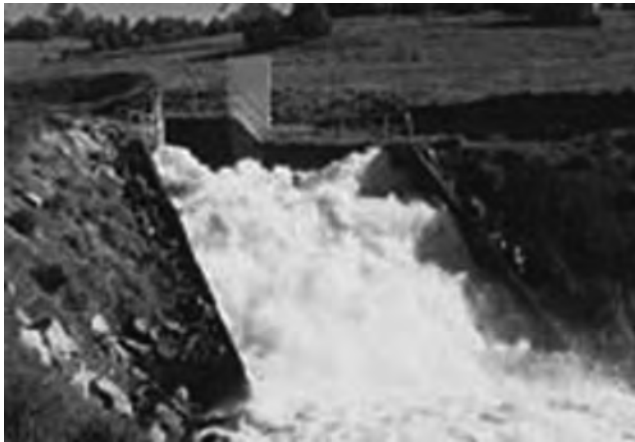
FIGURE 26.9 San Juan Chama Azotea tunnel outlet. (Courtesy of the U.S. Bureau of Reclamation.)
