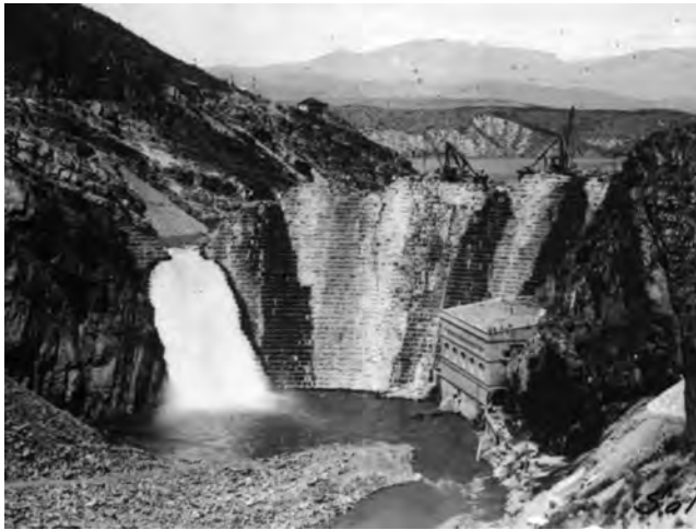
FIGURE 26.4 Roosevelt Dam under construction on the Salt River. (Courtesy of the Salt River Project.)
