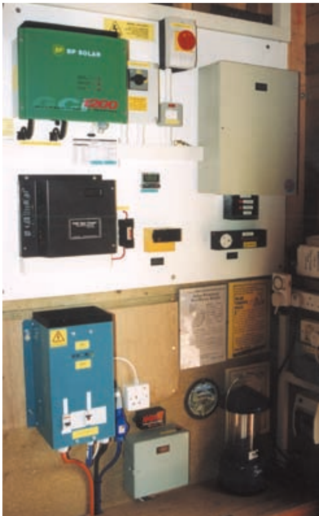
The grid-intertied BP inverter and related components, as well as the independent battery-based system, are housed inside the garden shed.
