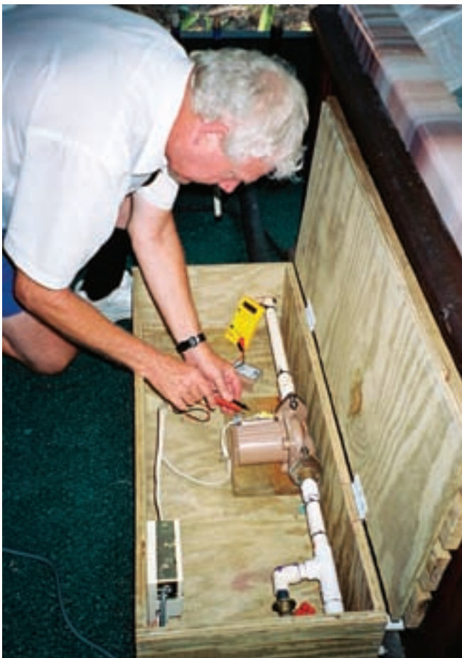
Bob uses a multimeter to test the voltage to the pump relay.
