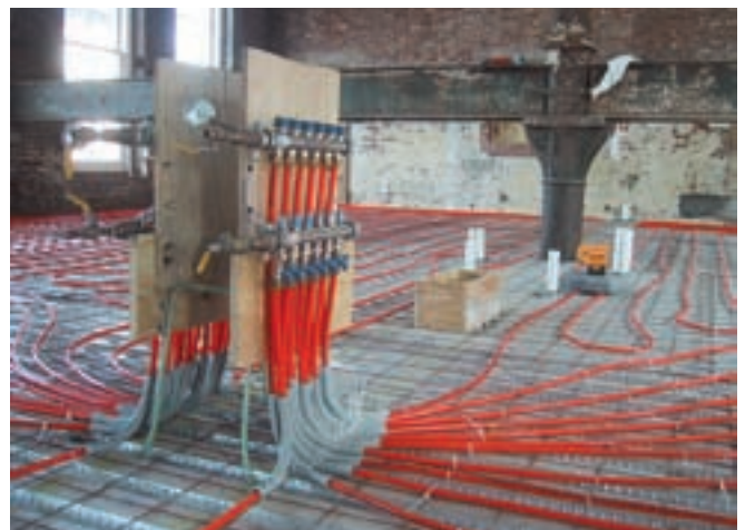
Installing the radiant floor heating throughout the building involved thousands of feet of PEX tubing.
