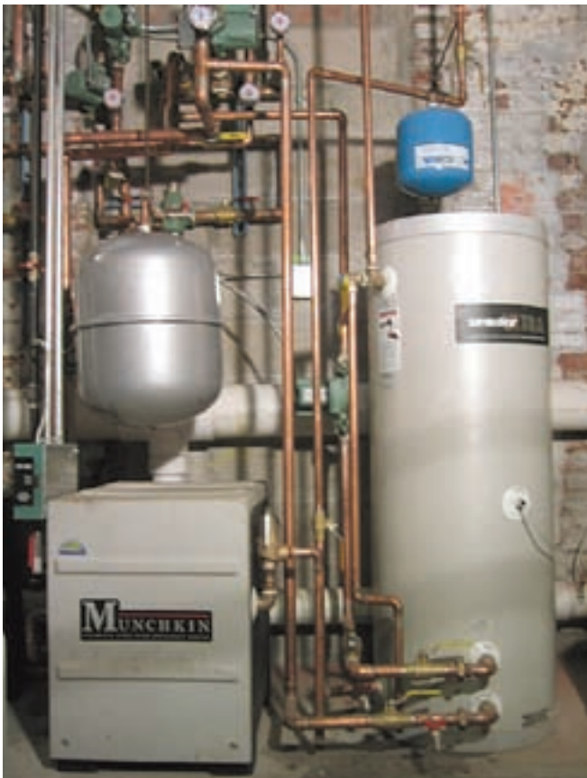
These Energy-Star-rated, condensing boilers provide energy-efficient heating for the icehouse's apartments.
