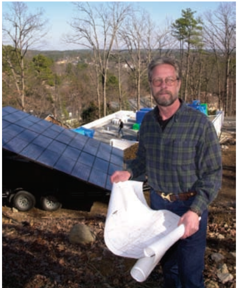
Author William Ball surveys the completed excavation and poured footings on Arkansas' first net-metered, solar-electric home. The trailed 2.4 KW PV array provides electricity for construction.
