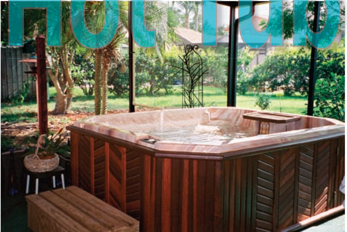
Bob and Barbara Owens' hot tub in their screen room, with the solar hot water system running. Water from the collector flows into the hot tub when the tub needs a temperature boost.
