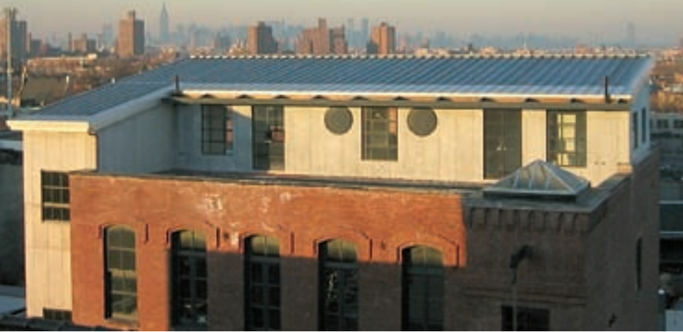
Seven kilowatts of Uni-Solar photovoltaic laminates cover almost the entire 1,200-square-foot area of the icehouse's rooftop addition.
