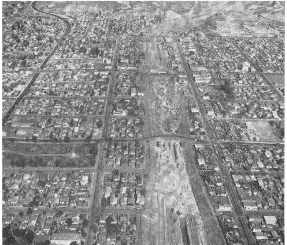
Construction on the Long Beach Freeway extension. This northward view was taken from above Olympic Boulevard.
