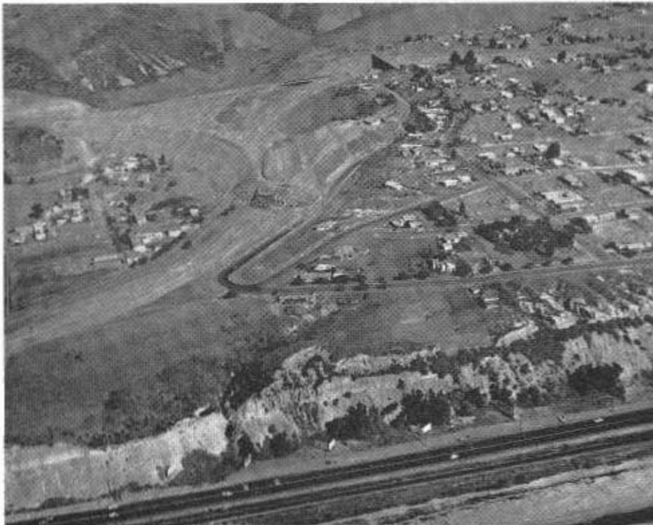
An interconnecting roadway is being constructed between U.S. 101 (foreground) and the San Diego Freeway (background) in the Capistrano Beach area. The view is eastward.
