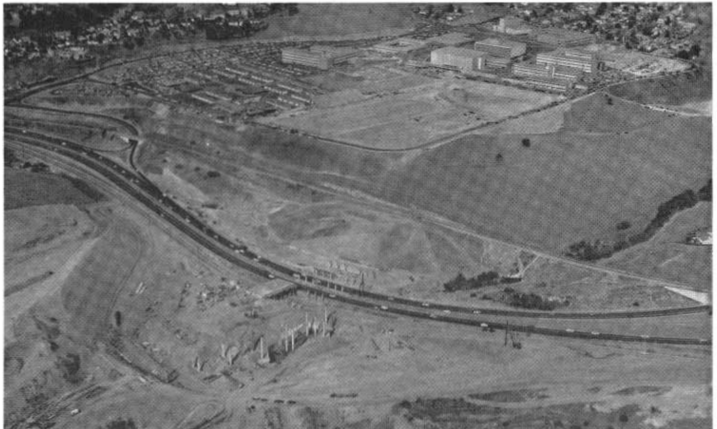
An aerial view northward showing construction work on the interchange which will connect the existing San Bernardino Freeway and the Long Beach Freeway extension. Los Angeles State College is in the background.
