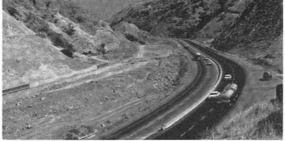
Considerable progress made on conversion of Grapevine Grade, US 99 in Kern County, to eight-lane freeway.
