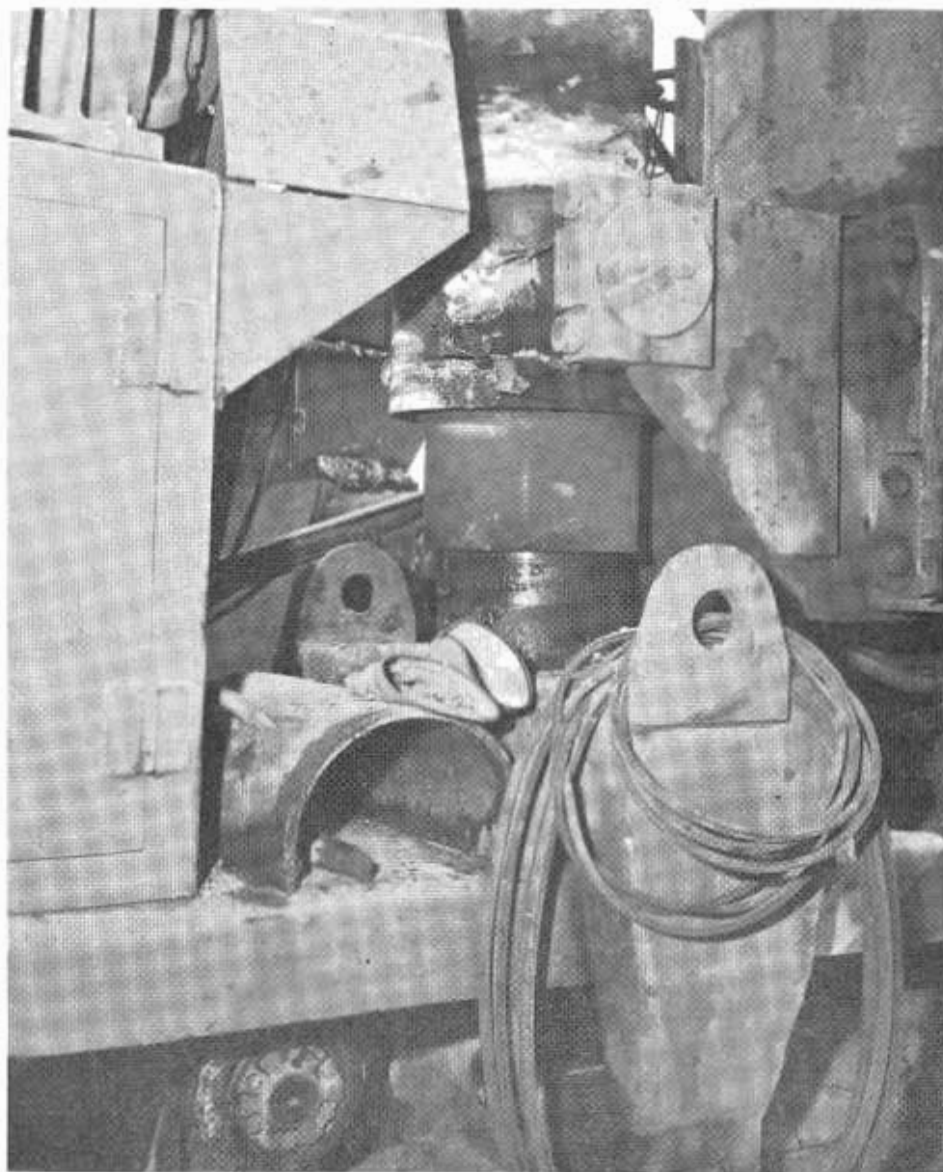
A close-up of the slip-form paver showing the right rear hydraulic ram in the center of the photo.
