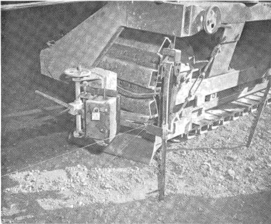
A close-up of the paver showing the left front elevation control probe passing by a stake with the steering control probe just behind the stake.
