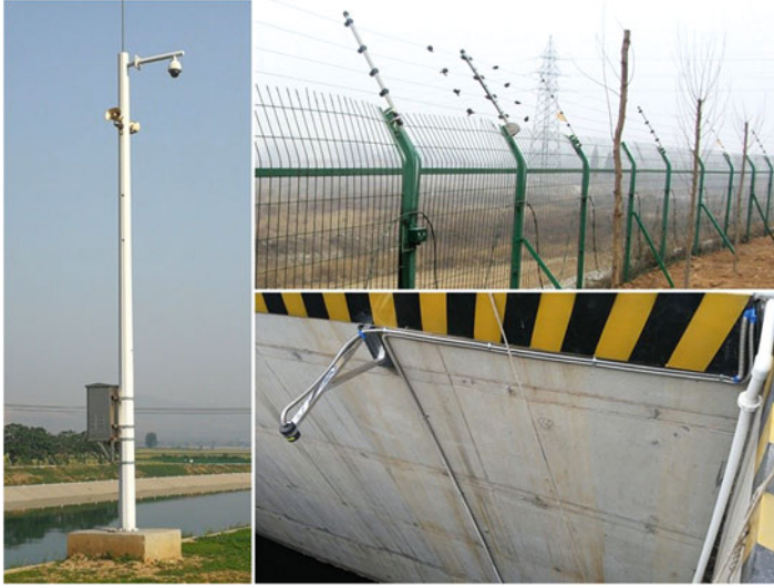
Fig. 1.10 Internet-connected sensors installed along the canal include video cameras (left), as well as intrusion detection (top right) and water level sensors (bottom right)
