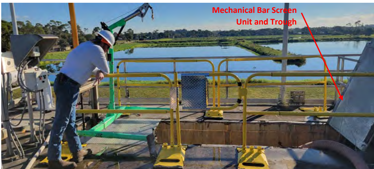
Annual Mechanical Bar Screen PM – Fall Protection Measures
