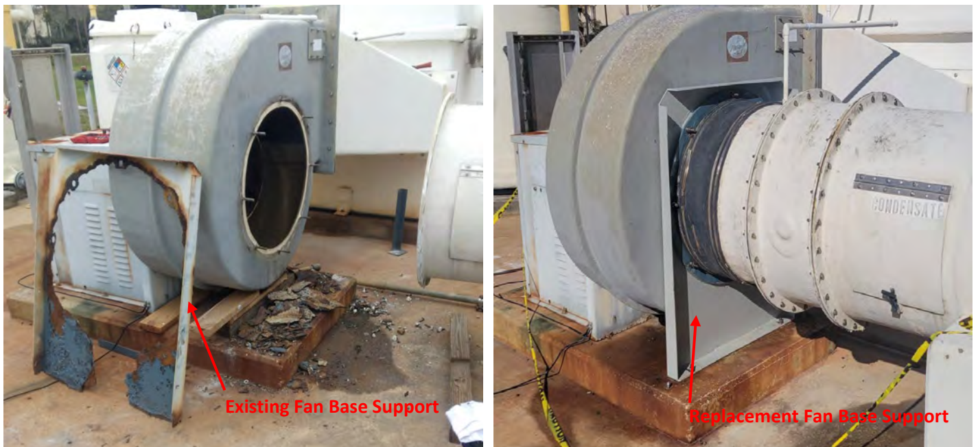
Sludge Tank Odor Control System – Before and After Repair Photos
