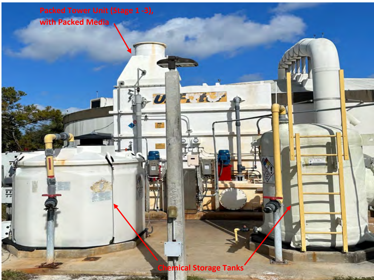
Sludge Storage Tank – Packed Tower Chemical Odor Control System
