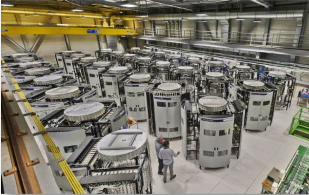
Figure 3. CERN SPS Thales solid state power amplifiers: 32 towers x 144 kW @ 200 MHz, combined in 2 x 2 MW amplifiers; in operation since 2021.
