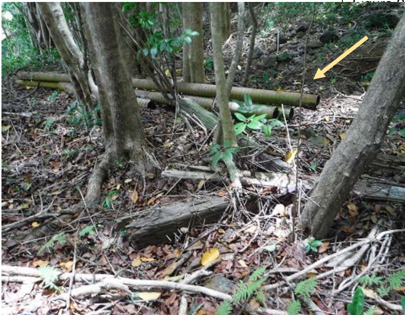
Figure 26: When removing abandoned pipes [arrow] workers should be alert for centipedes and other dangerous species inside or under.
