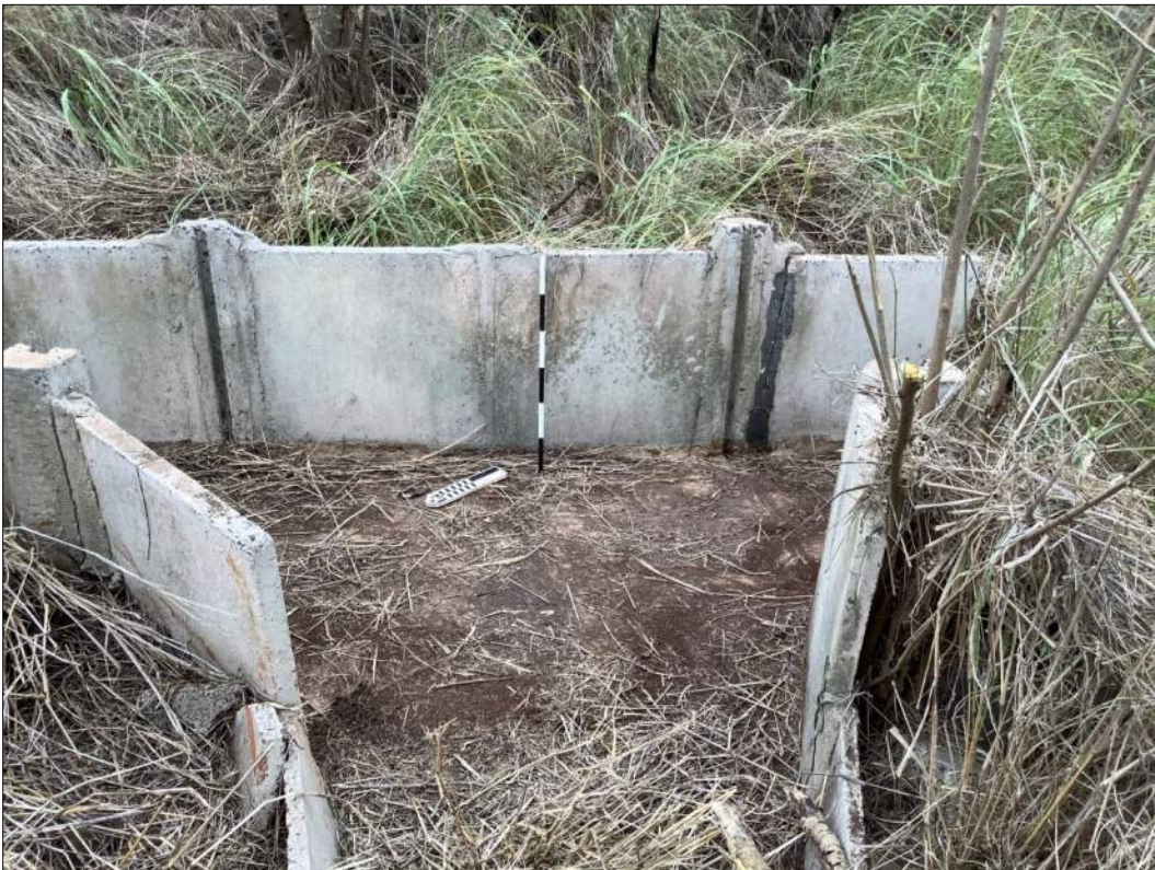
Figure 45. Site 7346 Feature 155-A, sluice at the intersection with Feature 155-B, view to the southeast.
