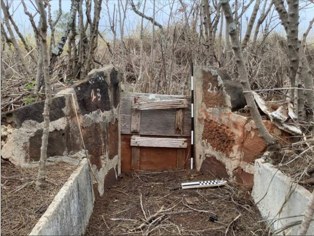
Figure 52. Site 7346 Feature 155-D, sluce gate at Feature 155-E, view to the west.
