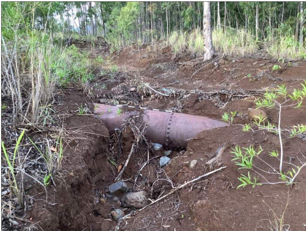
Figure 82. Exposed metal aqueduct pipe.
