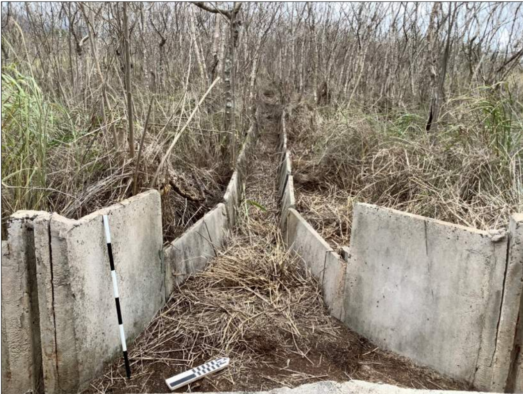
Figure 46. Site 7346 Feature 155-B, view to the northeast from the sluice at the intersection with Site 7346 Feature 155-A.
