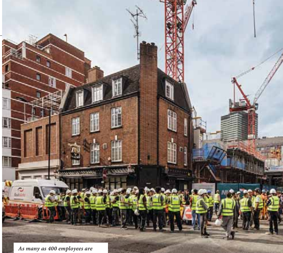
As many as 400 employees are working on the site at peak periods.
