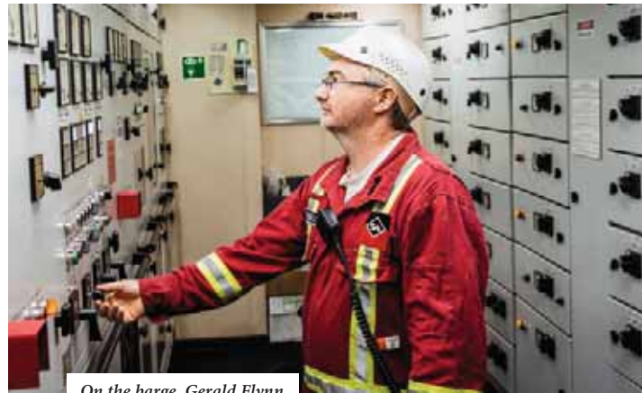
On the barge, Gerald Flynn controls the transfer of the raw material.
