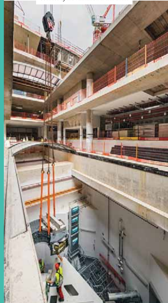
The concrete structure that houses the cyclotron was built on the building's fourth basement level because of the radiation it will emit.
