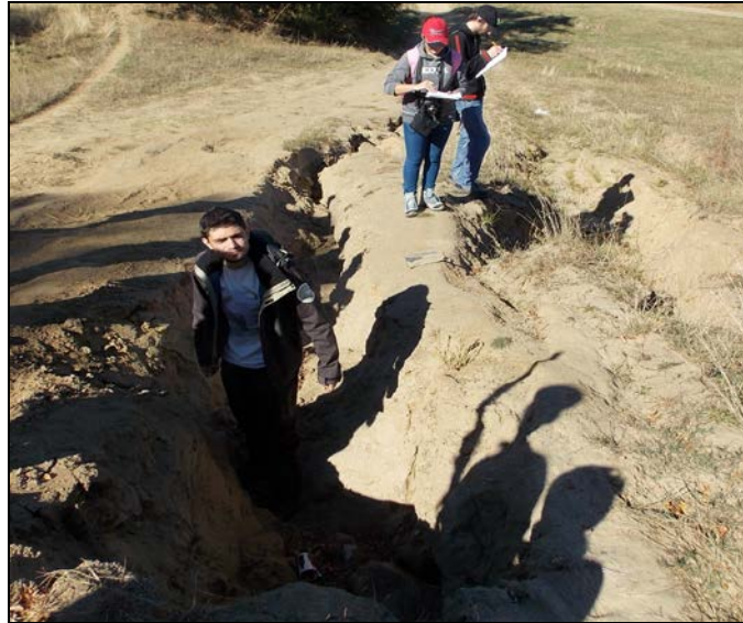
Figure 5: Deepening and upstream extension of the runoff channels through the processes of suffusion and regressive erosion and the evolution into more advanced form.
