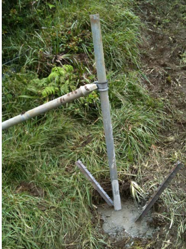
Reinforced Poamoho footing: 8' round post driven to 4' with two 7' t-posts for stability driven to 6' all tied together with 150 lbs of concrete (dry weight).
