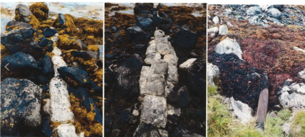
Figure 7 - North Uist shore end, showing exposed cable
