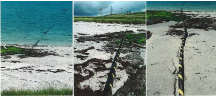
Figure 5 - Eriskay 1b (towards Barra), showing exposed in-service cable
