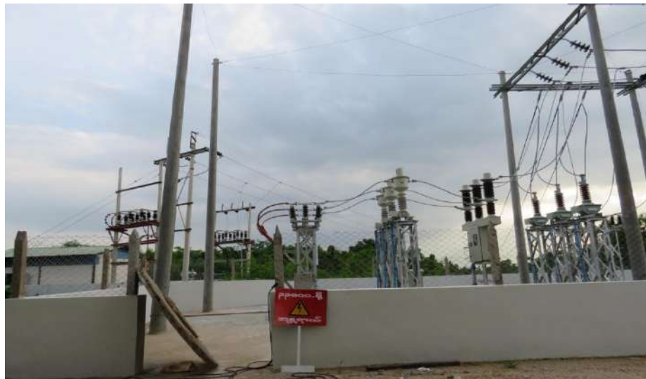
Figure-18: Electricity sub station
