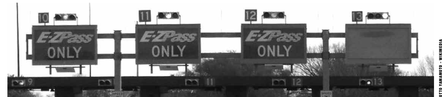
A toll gantry on the Pennsylvania Turnpike.
