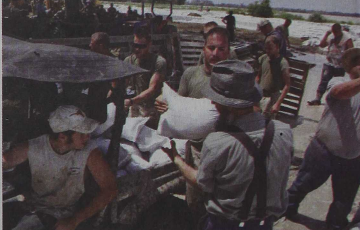
Marines and sailors work together with locals to reinforce the levees. Cpl. Jason D. Mills
