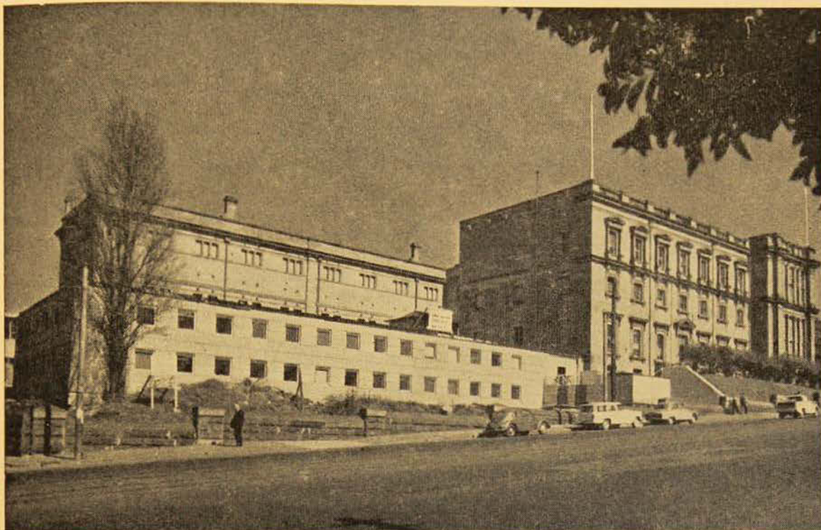
The completed two floors of the new six-storey wing being built at the Museum. Construction of the remaining four floors and a public cafeteria on the roof has commenced, and will be completed in March, 1962
