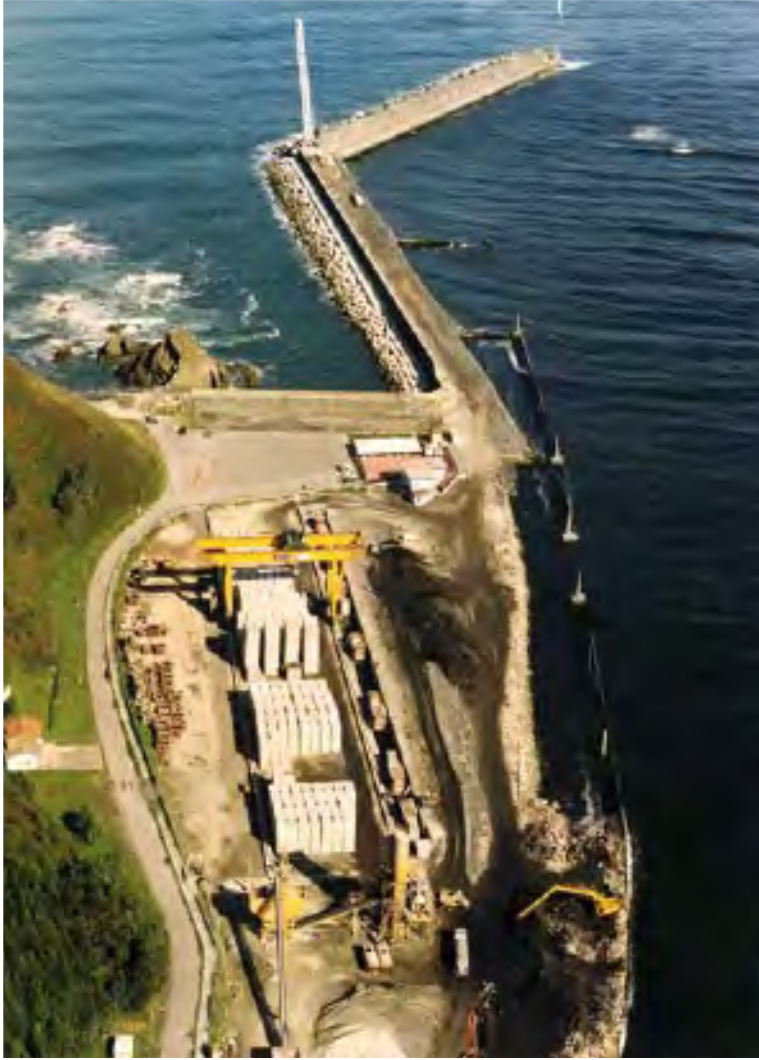
The San Esteban de Pravia harbor is linked to the history of Obrascón. Almost eighty years separate one of its first contracts for dredging the harbor's access channel and the channel restoration works in 1998, when this photo was taken.
