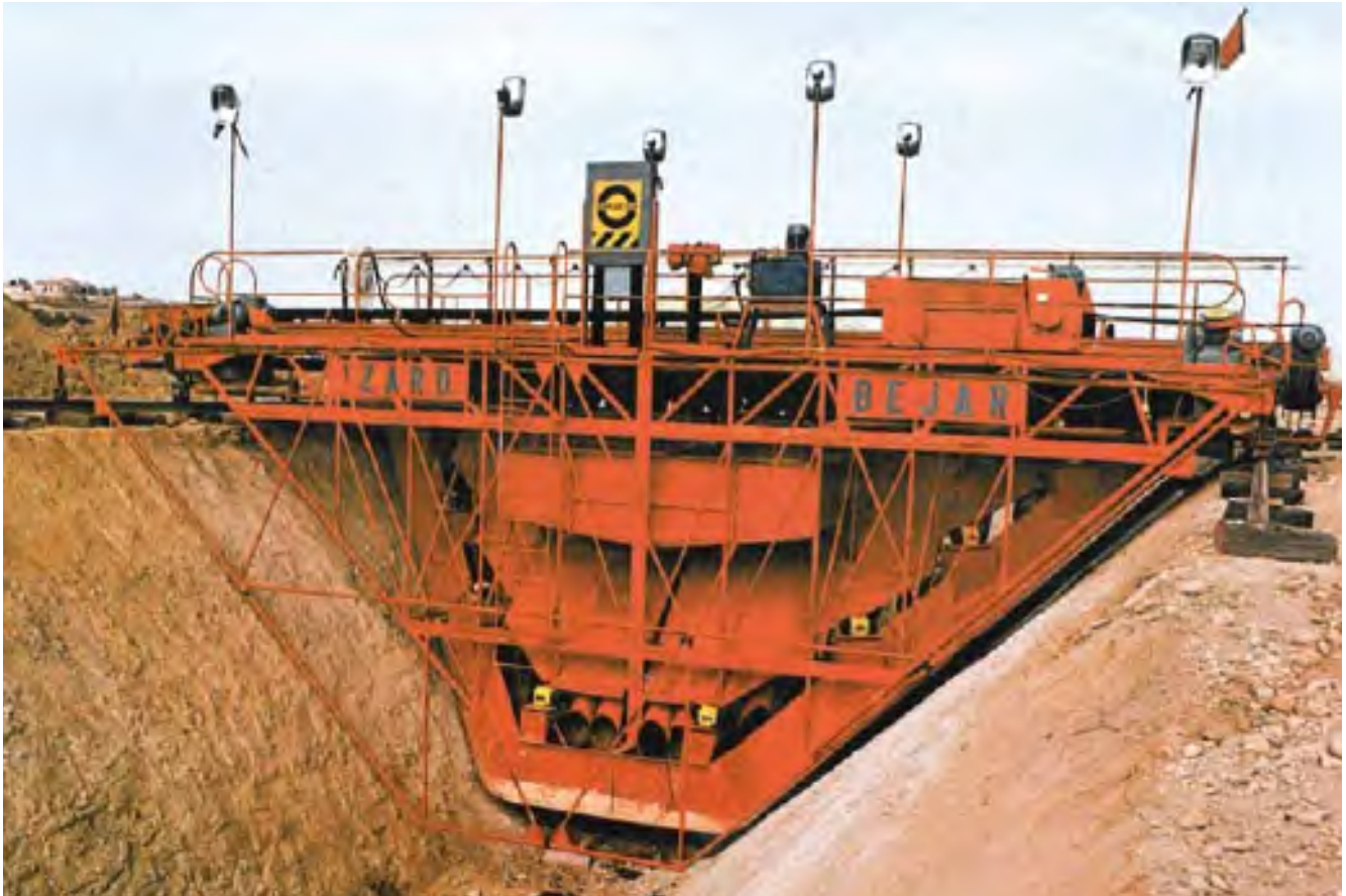
An Obrascón motor-driven sliding formwork used in the construction of the Crevillente Canal, one of the major projects undertaken in the eighties.
