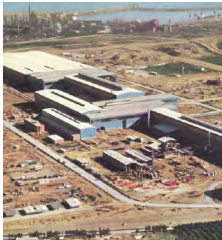
Obrascón changed hands in 1973. Altos Hornos de Vizcaya (AHV) purchased it for building the 4th integrated steel plant in Sagunto, the construction of which is shown above.
