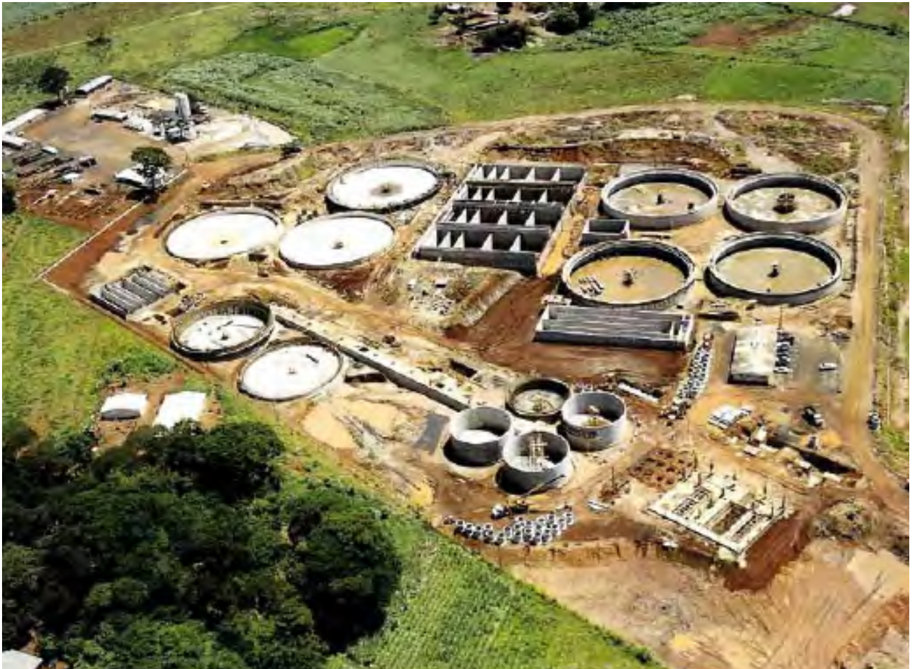
The construction of the Riberao Preto sewage treatment plant, in Brazil, has been one of the most significant projects connected with the “water and environment” area, as it was designed for providing service to 600,000 inhabitants.
