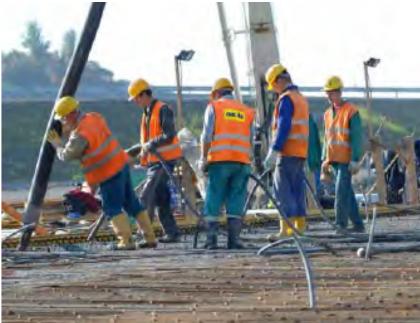
OHL's most relevant European investment in 2003 took place in the Czech Republic. OHL purchased a controlling interest in the construction company ZPSV-ŽS Brno (OHL ŽS at the present time). It was the first of the positions taken up in the markets of Central and Eastern Europe. Above: OHL ŽS workers on a Central European railway.
