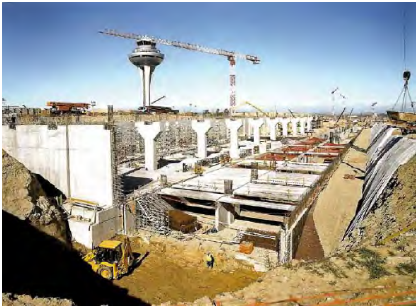
During 2001, 35% of the total budget contracted referred to building construction. The Satellite Building of the new Terminal 4 of the Madrid-Barajas airport, built by OHL for Aena, ranks among the most outstanding awards.
