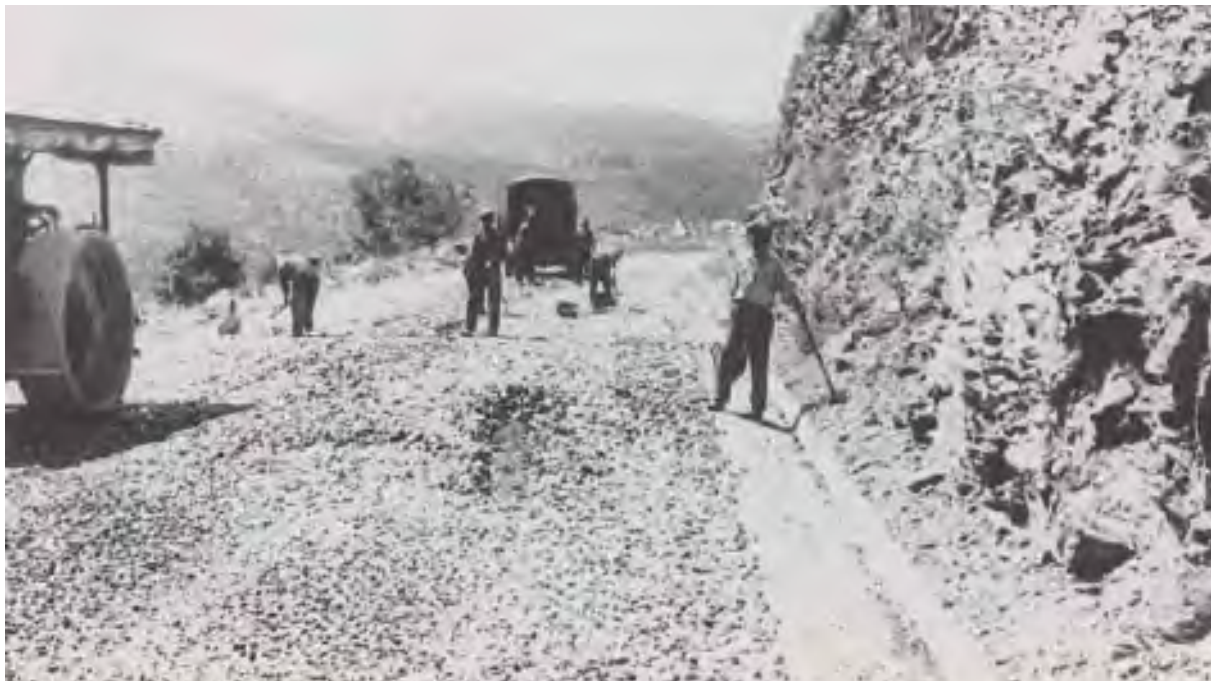
The road modernizations plan undertaken in 1951 enabled the asphaltting of many old stone paved roads and initiated the improvement of road connections. In the photograph, work on a stone paved road.
