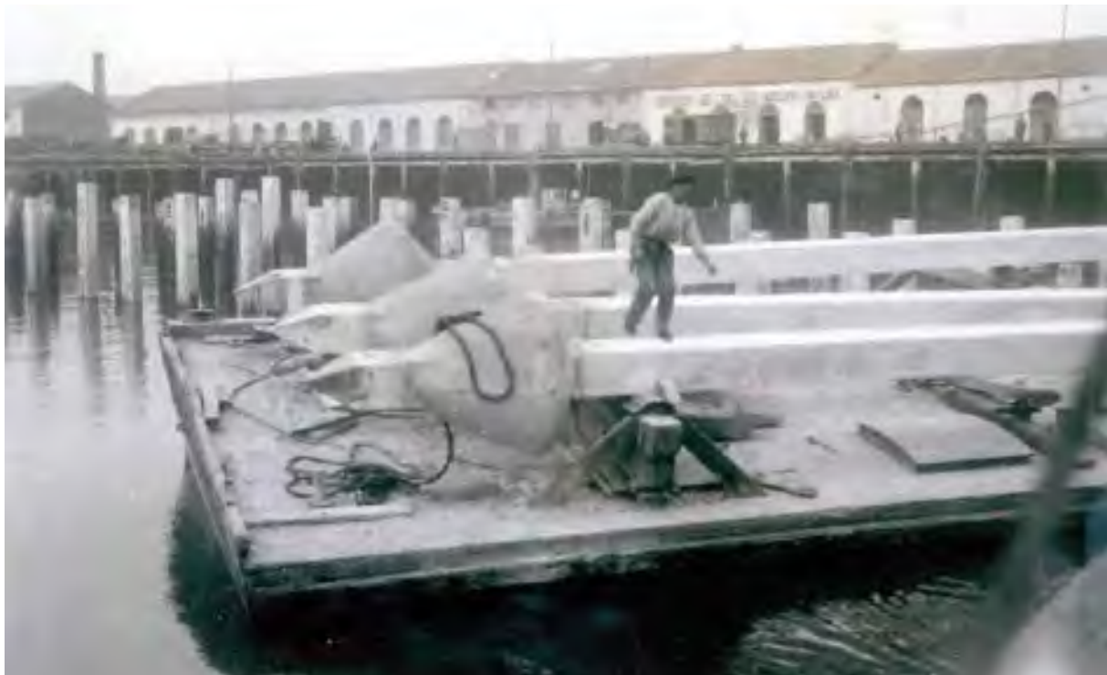
Driving of prefabricated concrete piles at the Port of Santander, a project performed by Obrascón in 1930.
