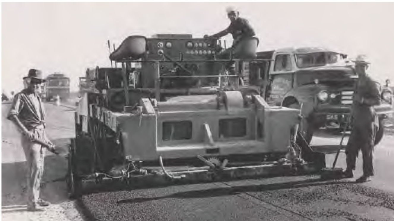
The 1950 plan for the modernization of Spanish roads gave strong impetus to the quality of these infrastructures, as well as to asphaltting machine technology. In the photo, the latest model of a self-propelled Alfelder spreader, recently imported from Germany.
