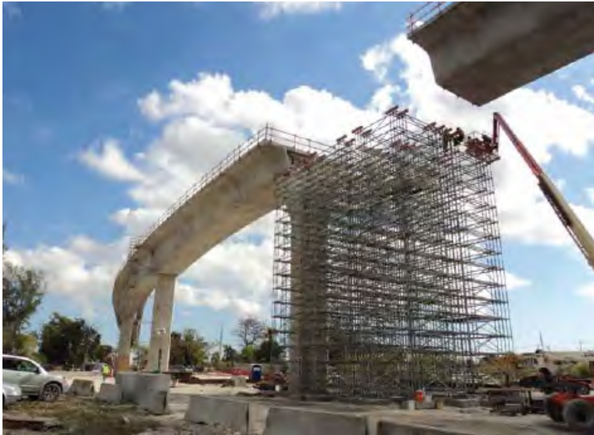
Optimizing the safety of employees in construction processes is one of the priorities of the R&D&I of the sector. In the photo, OHL construction work on the Miami Metronail line to the city's airport.
